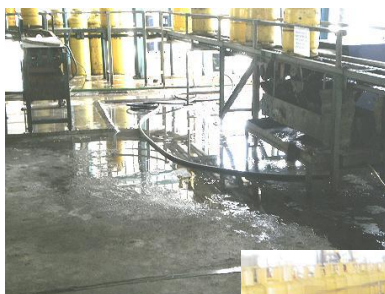
Before OSDEC BIO-LUBE application – Wet and slippery
